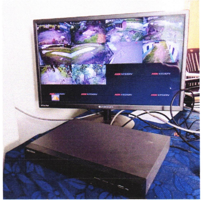
CCTV MONITOR AND NVR
