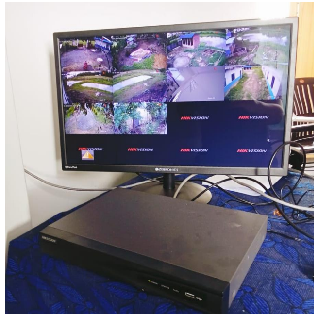
CCTV MONITOR AND NVR
